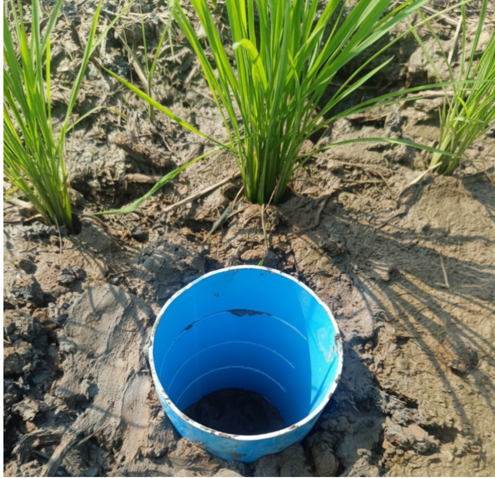
Figure 3: Installing a perforated PVC pipe into the field to monitor the subsurface water level
